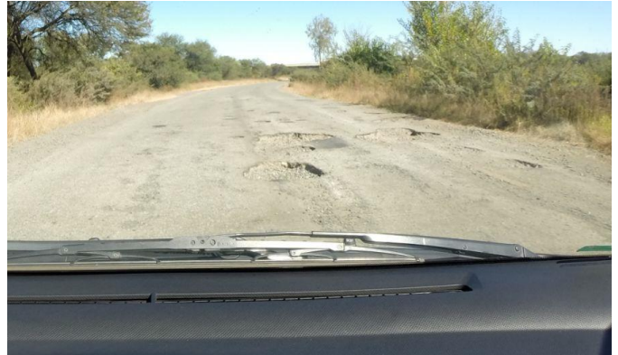
Fig. 1. Example of potholes in a road
