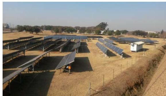
Figure 2: Aerial Photograph of ERIC Solar PV Facility
