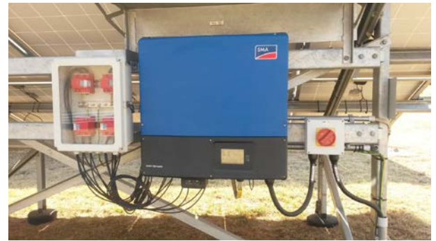
Figure 5: Typical Multi Crystalline Configuration for the Inverter at ERIC
