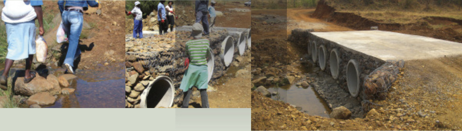
Access for rural communities in the Albert Luthuli Municipality in Mpumalanga before (left), during (centre) and after (right) infrastructure interventions
