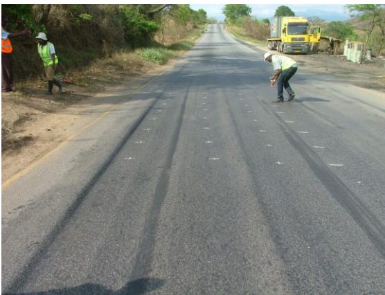
(e) Rutting on Mikumi-Iyovi road section
