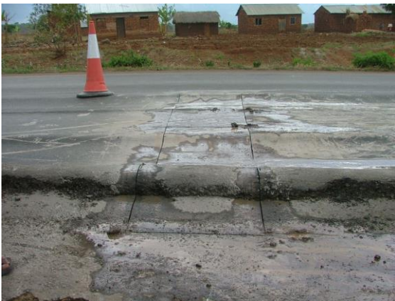
(g) Rutting on Makambako-Mbeya road section
