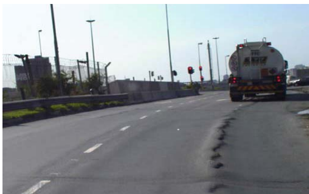
(a) Severe rutting on the South Coast Road section prior to rehabilitation
