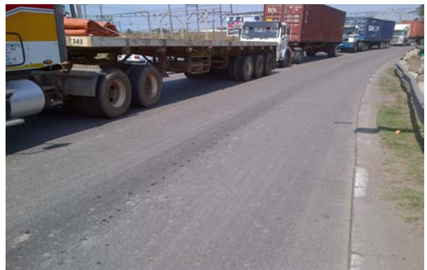
(b) Condition of the South Coast Road section two years after rehabilitation
