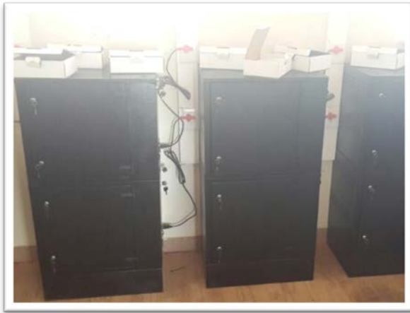
Photo 1-9: Secure charging station used in Phase 1
