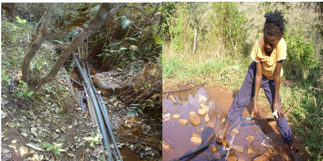
Figure 2: Pipes connected at the spring sources (left) and water being collected from a pipe (right)
