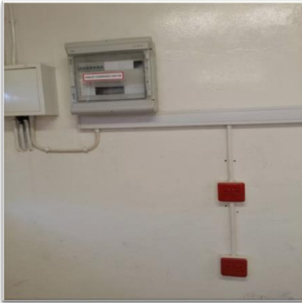
Photo 4-5: Data and electrical reticulating and for charging the tablets
