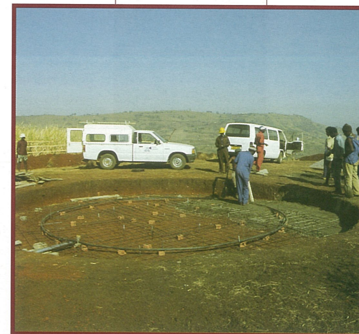
The CSIR-designed water supply scheme at KwaNyuswa has demonstrated the success of community involvement in projects.
