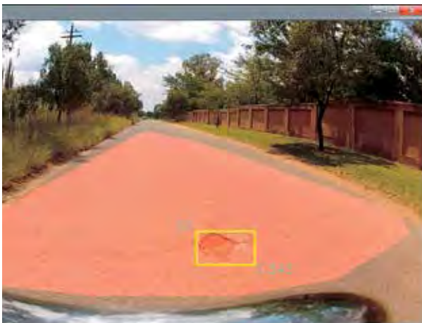
Automated video analytics detecting the road and classifying a pothole.
