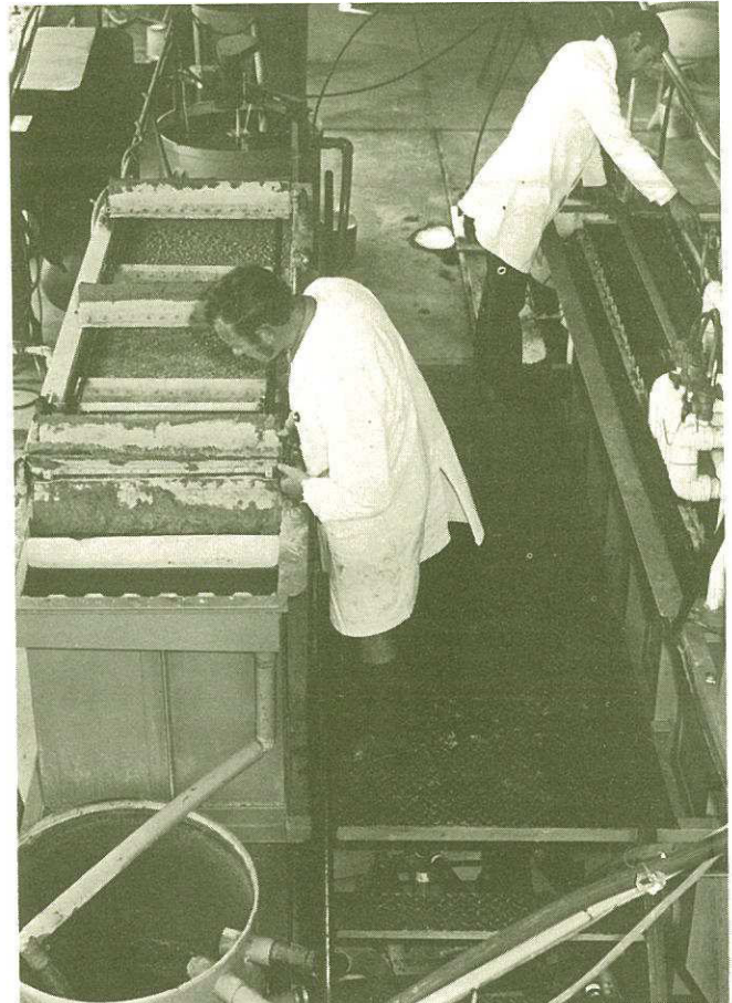
The LFB process is based on chemical pre-treatment of raw or primary clarified sewage with lime, followed by biological processes and further physical-chemical treatment. The stage shown here is biological treatment which follows chemical pre-treatment.
