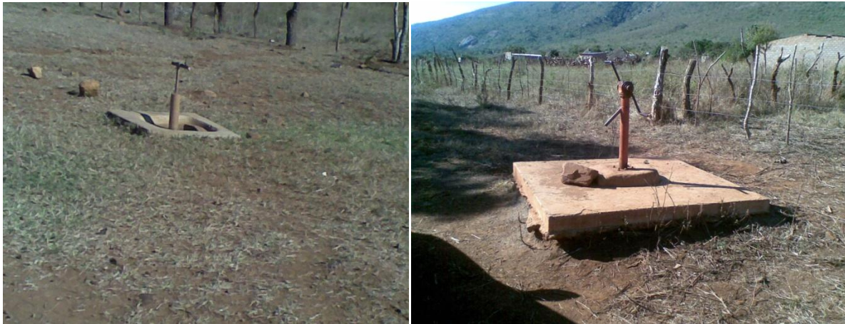
Figure 17: A photo of a communal standpipe (left photo) which has not been working for a almost three weeks, and a handpump(right photo) which has not been working for about 12months in Thambonkulu village
