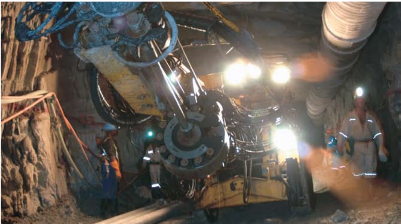
Rockfalls are a life-threatening reality in mines. An in-stope measurement system for underground sensing and communication, which also includes a number of sensors to gauge the condition of the roof, was developed by the CSIR.
