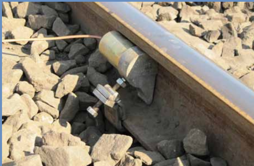
Custom ultrasound transducer for rail break monitoring, attached to the Sishen-Saldanha heavy freight railway line.
