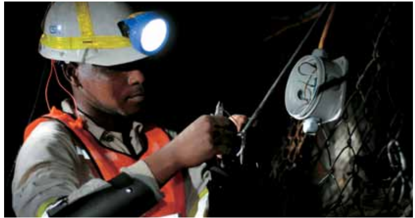
CSIR electrical engineer, Josias Nonyana, installs a connector to wires from a data logger, which connects to a geophone – an instrument used to measure seismic velocity. All collected data from the geophones are aggregated on the data logger. The data logger sends data to a server at the surface.
