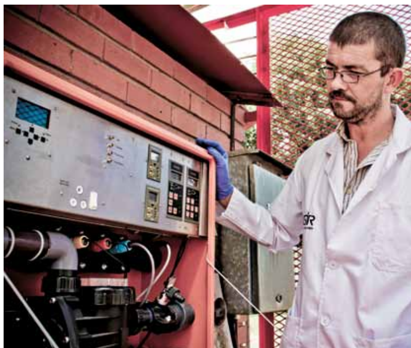
The CSIR's Calie Adlem inspecting a remote monitoring system installed at a water treatment plant.
