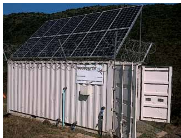
Various renewable and alternative energy supply options were investigated for the communal water stations. Solar power, as seen at this communal water station, with diesel generators as back-up was found to be the most suitable.
