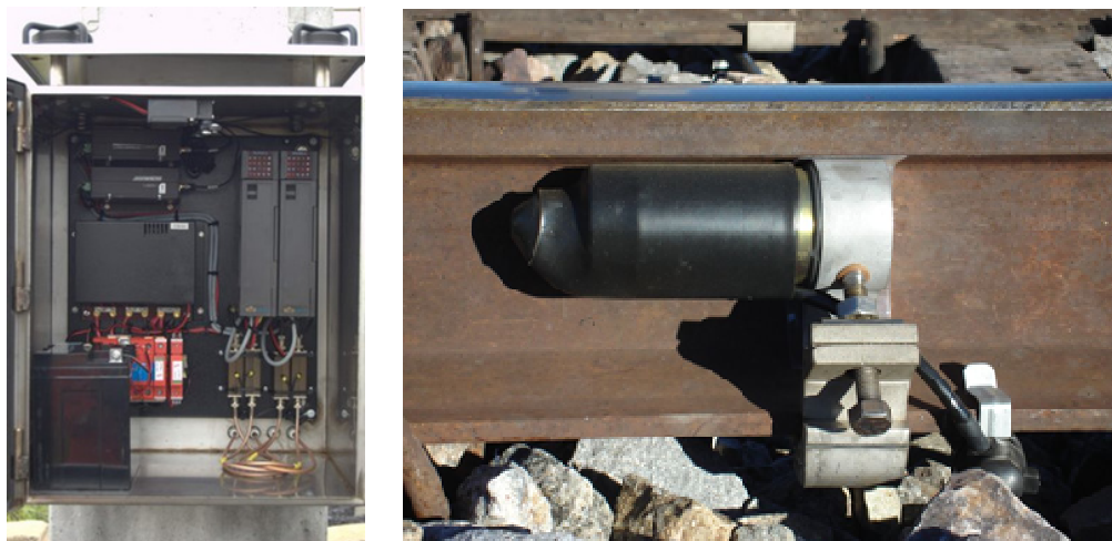
Fig 3. Transmit electronics and installed ultrasonic transducer [19]
