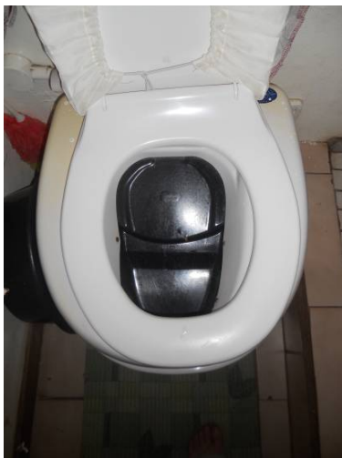
Figure 2: Example of UDD toilet in Hull Street (Source: CSIR, 2011)
