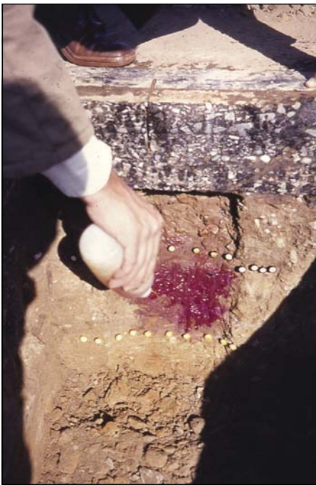
Photo 19 Fully carbonated and relatively weak upper cementitious subbase layer directly underneath the recycled asphalt base layer, resulting in a "sandwich" structure of a weak upper subbase on the N3 at Van Reenen's Pass (De Beer 1985)
