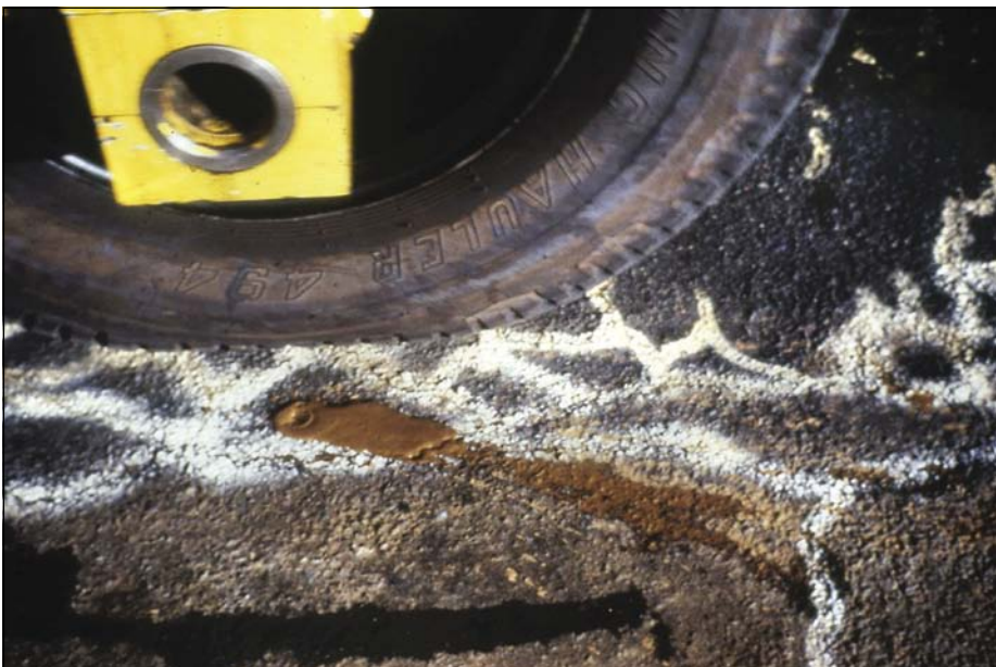
Photo 22 Signs of pumping from the cementitious base layer during a wet HVS test, after crushing in the dry state (De Beer 1990)
