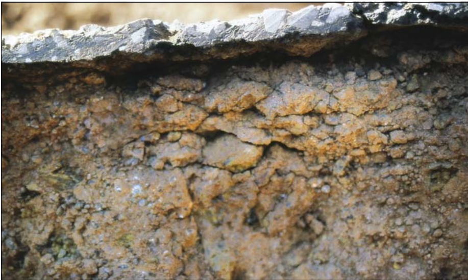
Photo 21 Crushing (dry condition) of a lightly cemented base layer as a direct result of HVS trafficking (De Beer 1990)
