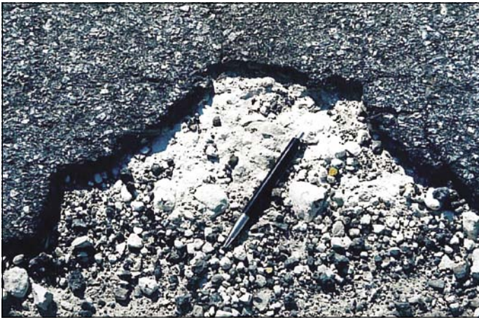
Photo 26 Typical signs of crushing failure in a pothole in a cementitious base pavement
