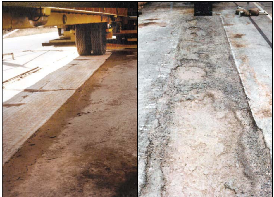
Photo 17 Failed HVS test section of a cemented base pavement (with 25 mm weak layer at bottom of 80 mm cemented base) after wet test at Hornsnek, Road P30, in 1985 (Opperman 1984)
