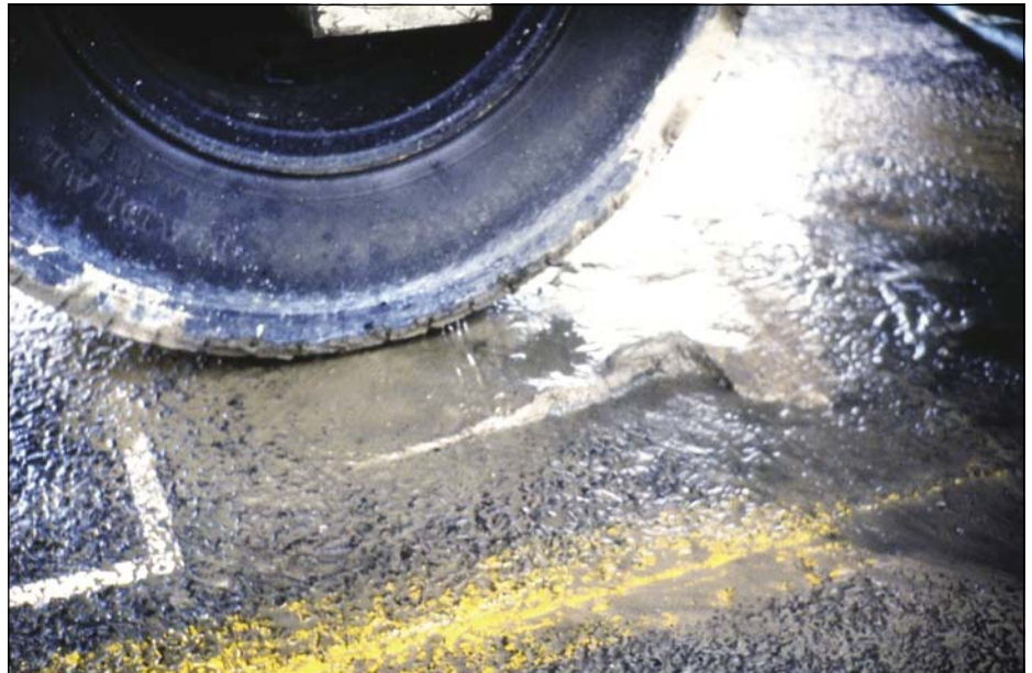
Photo 20 Pumping of fines during HVS testing from a strongly cemented (C2) base pavement (Road MR27) (Rust 1987; Jordaan 1988)
