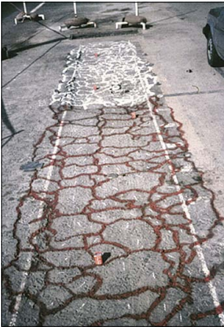
Photo 18 Crack pattern on recycled asphalt base layer on Van Reenen's Pass during HVS testing in 1985 (De Beer 1985)
