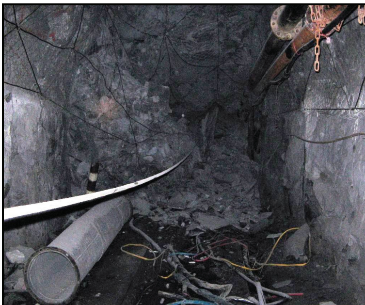
Figure 13. Extensive damage at the 1973 X/Cut due to EventID17700
