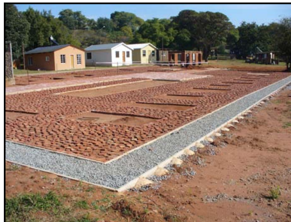
Figure 8 View of the Sanitation Technology Demonstration Centre under construction (Photograph taken by CSIR, 2010)
