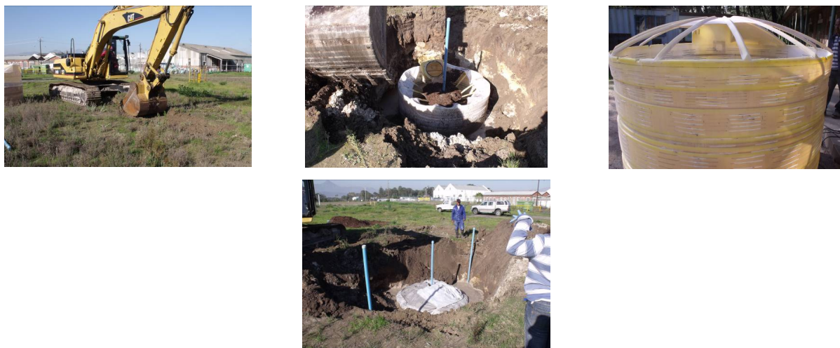
Figure 5. Digging and emplacement of tank used for carbon source during the experiment.
