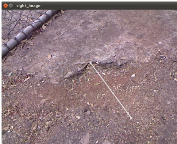
Fig. 4. Pothole width measurement.
