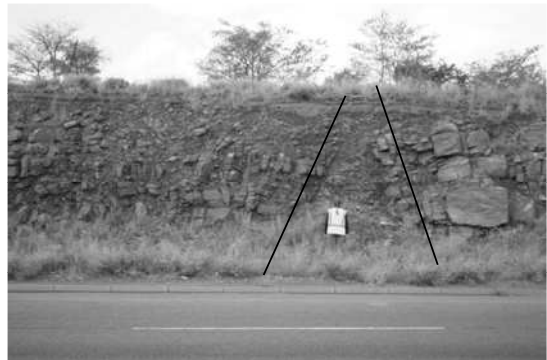
Dykes – Very weathered
