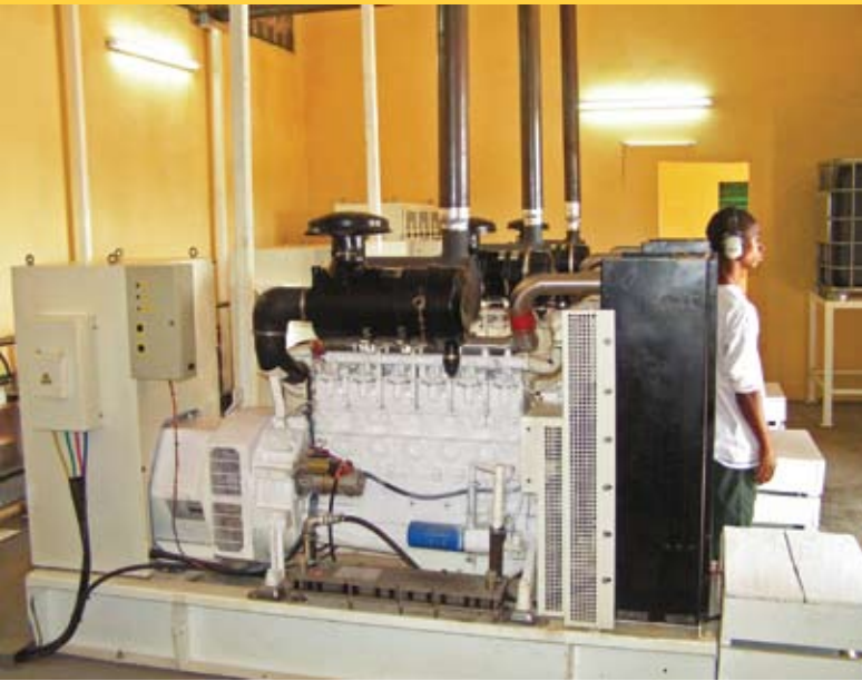
An operator stands in front of a bank of 100KW diesel generators designed to run on either diesel or jatropha oil at the Mali Folkecenter in Garalo, Mali. (Photo by Graham von Maltitz)
