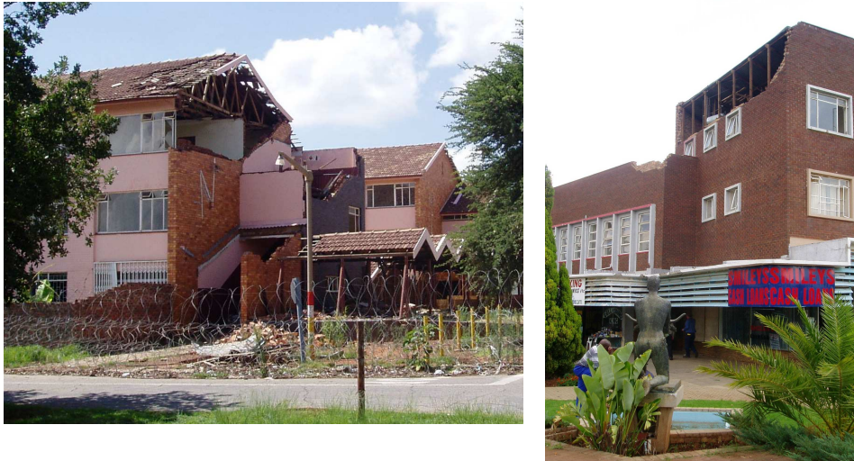
Figure 22. Damage to buildings in Stilfontein following a magnitude 5.3 mining-related earthquake (from Durrheim et al., 2007)
