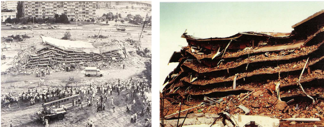
Figure 23. Damage to a block of flats in Welkom following a magnitude 5.2 mining-related earthquake (no fatalities)
