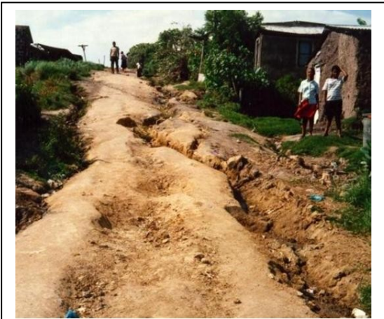
Eroded township street
