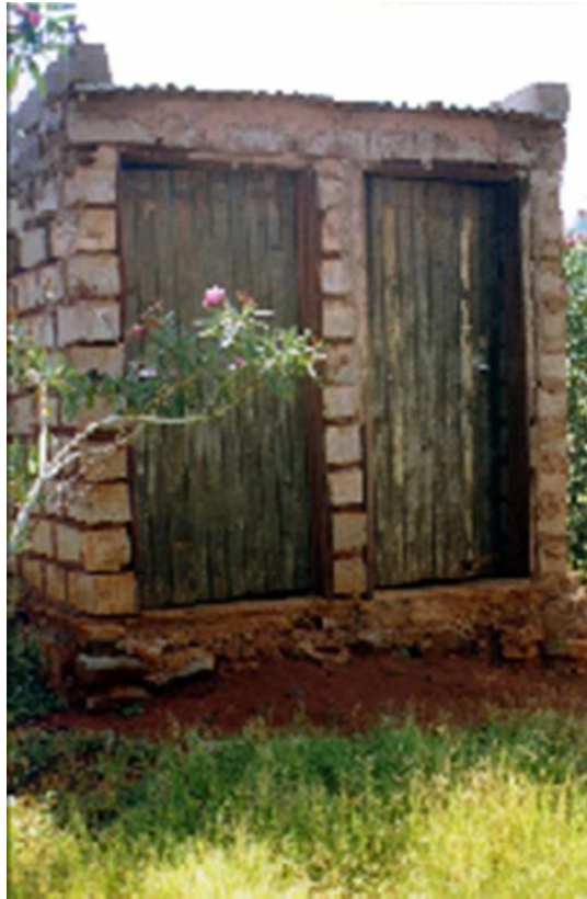
Sanitation also has to provide for cultural requirements, for example by providing male and female facilities. Example: Mathabatha Source: C. du Plessis, CSIR
