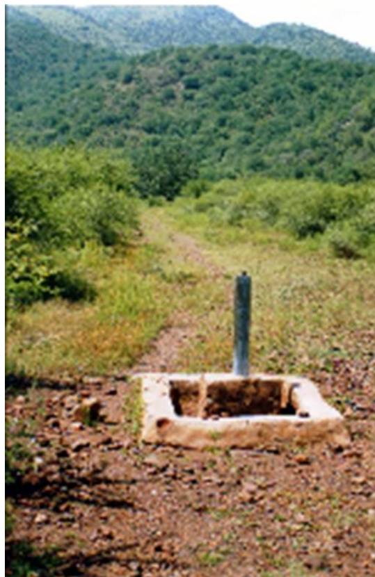
Rural water supply: Stand pipe in Mathabatha, no longer in use.
