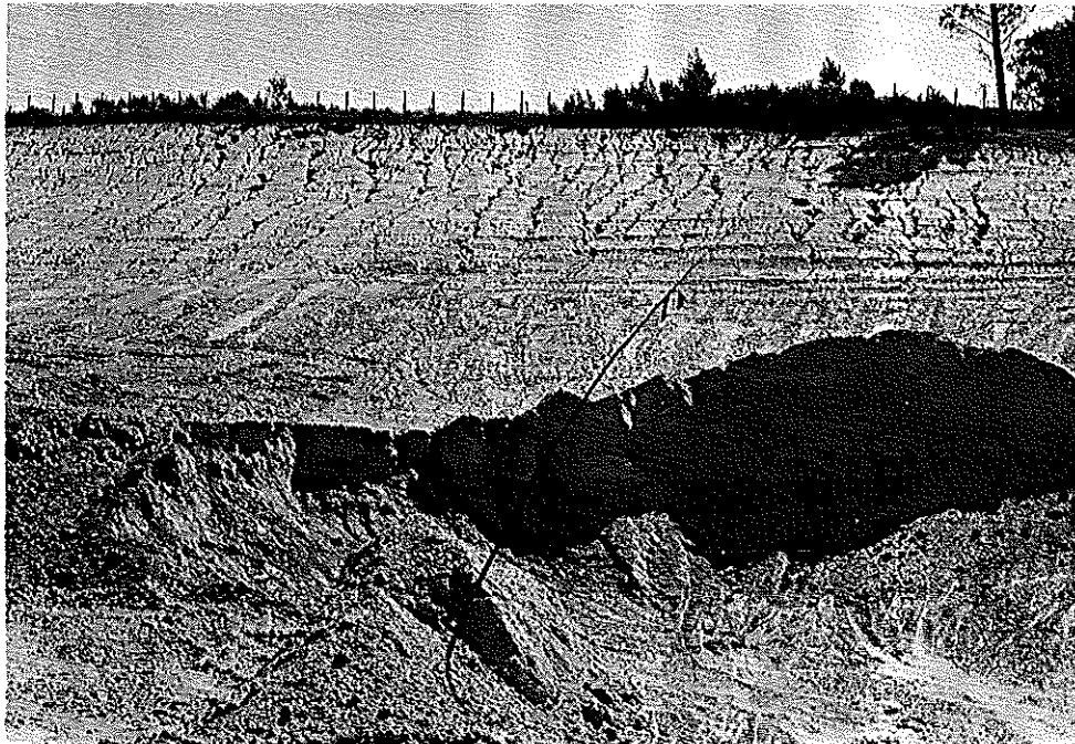
FIG. 5: Road construction adjacent to the Wolwe River showing one of the sources of sediment which enter Swartvlei following heavy rain (IFWS: 83-03-08).
