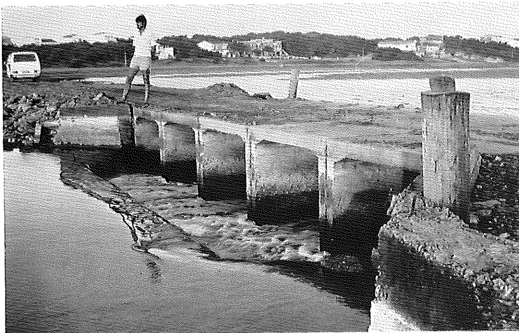
FIG. 24: Central section of the Seekoei Causeway showing existing culverts which are insufficient to accommodate adequate water circulation. The water level downstream (RHS) of the causeway was significantly lower than upstream (LHS) in this photograph due to the mouth having just been breached. (ECRU: 86-01-19).
