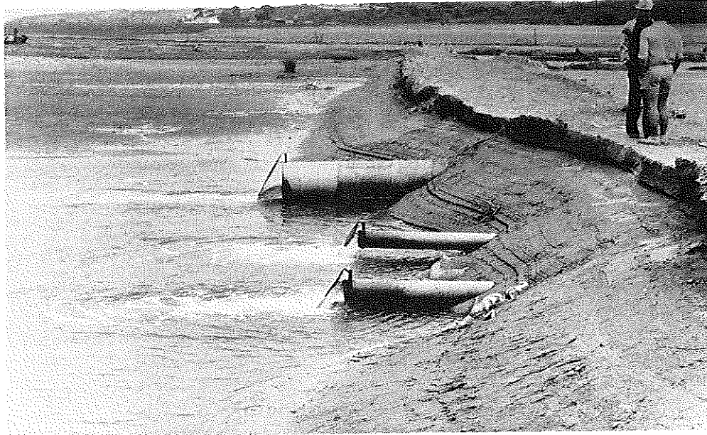
FIG. 26: Illegal earth weir built across the Gourits River about 1,5 km upstream from 'Die Eiland' (H. Lüttig, DWA, 87-09-14).
