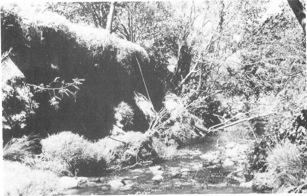
FIG. 33: Shallow-rooted trees, particularly alien Acacia spp., give little protection to the river banks and are often uprooted during spates. (Photo: WCRSC).
