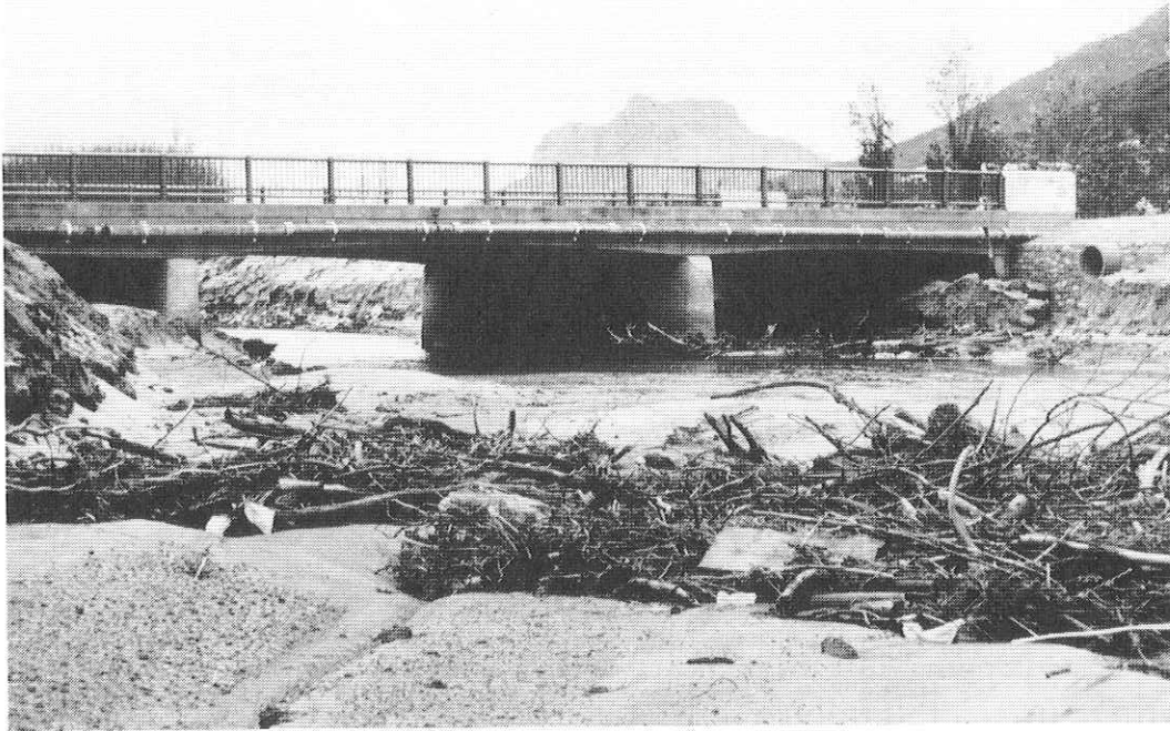
FIG. 35 : Silt and debris deposited under Victoria Road bridge after the flood in June 1983. (Photo: S Grindley).
