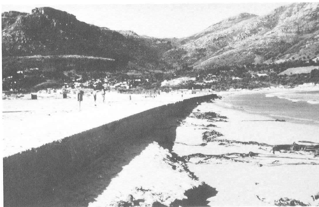
FIG. 40 : Sea-wall west of the river mouth with an artificially hardened parking area behind it. (Photo: ECRU, 82-04-19).
