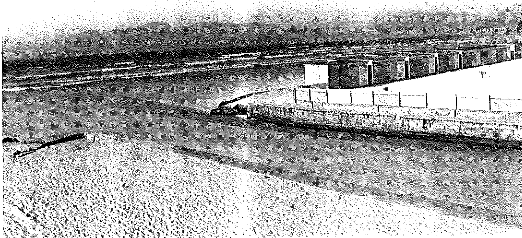
FIG. 10: The canalized mouth of Sandvlei. Note the collapse of the concrete walls at the seaward end.
