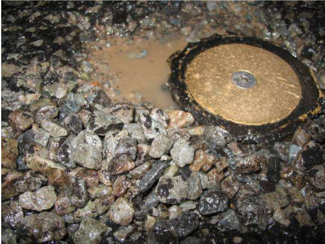
FIGURE 3 Indication of stripping of HMA due to wet HVS test.
