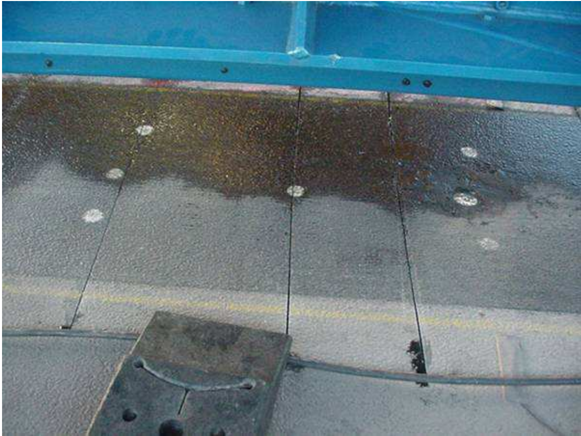
FIGURE 5 Indication of slots sawn into surfacing to allow water penetration through impermeable surfacing.
