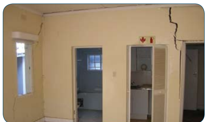
Fig. 2: Some evidence of the structural damage that can be observed at the 13th Avenue property.
