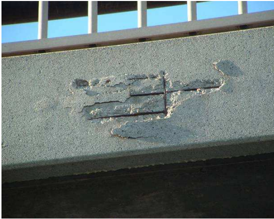
Figure 2: Spalling on side of deck due to inadequate cover over reinforcing
