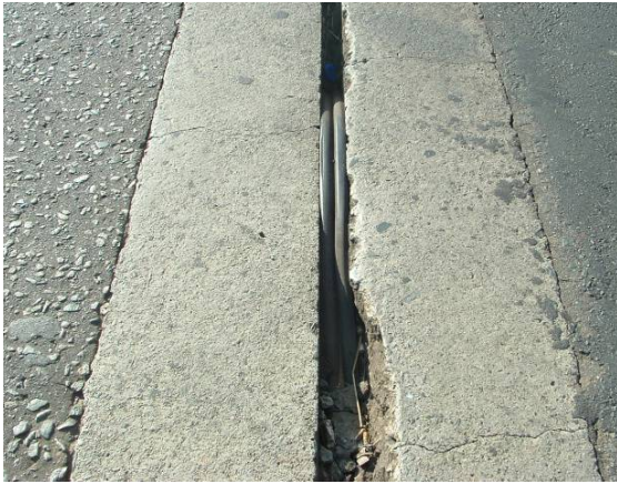
Figure 4: Failed elastomer element in expansion joint
