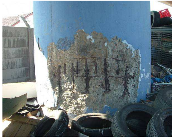
Figure 3: Spalling on piers
