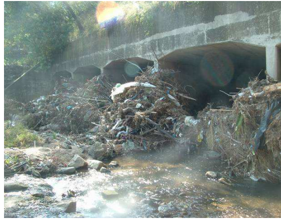
Figure 5: Accumulation of debris against piers
