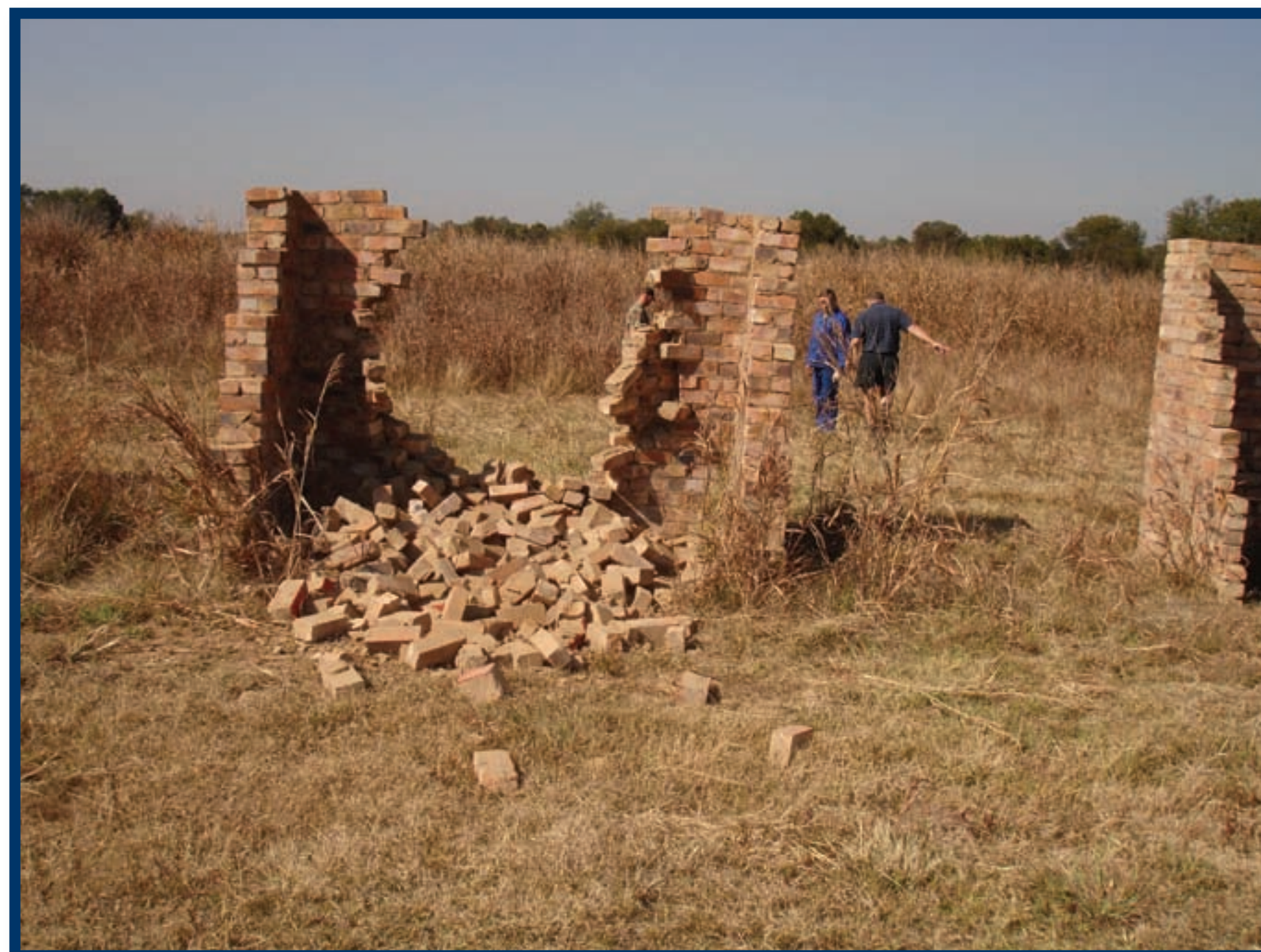
Figure 1. Damage to double brick wall (3 m x 2 m)
