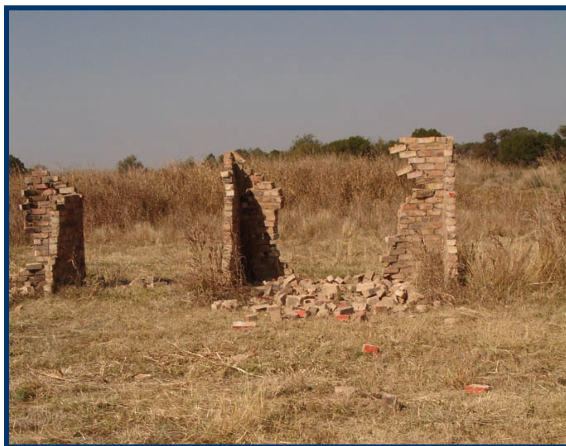
Figure 2. Damage to single brick wall
