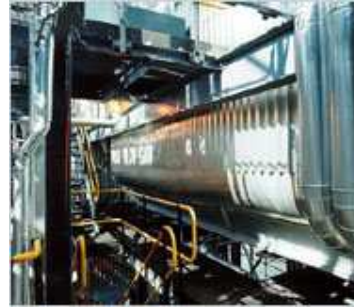
A boiler after a fluidised bed
