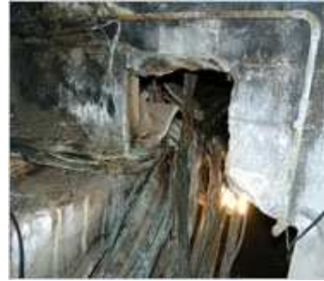
Destruction left by the underground fire
