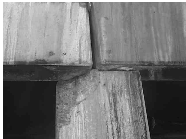
Fig. 4. Spalling of deck beam seating on top of pier trestle beam (B2167).
