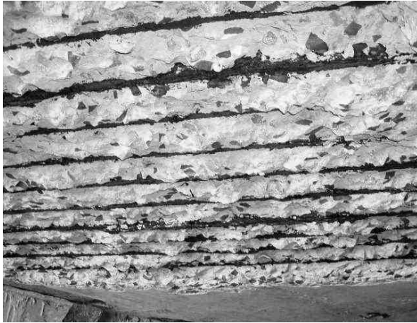
Fig. 1. Delamination of large areas of concrete at soffit of culvert top slab (C10447).
