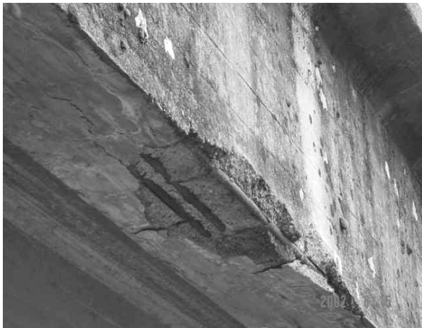
Fig. 3. Spalling of concrete at deck beam soffit (B2983).
