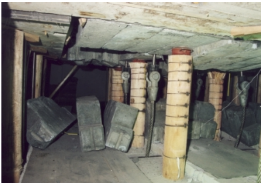
Photograph 5.2 Test # 4, all roof blocks collapsed except those directly above the elongates.
