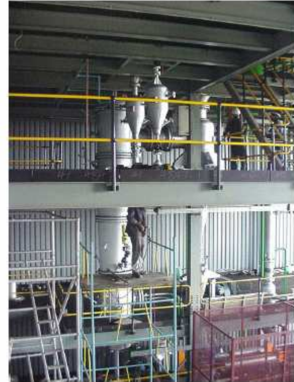
ESKOM 150kW Pilot Plant
