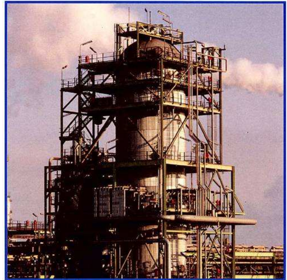
The Sasol Advanced Synthol reactor
