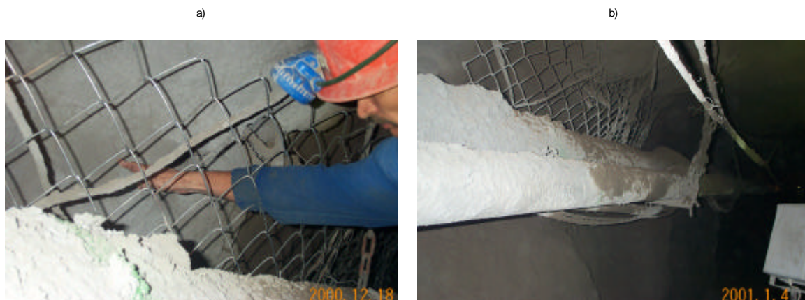
Figure 15: Areas where mesh could not be pinned to the shotcrete.
