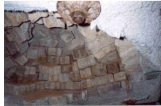
Figure A.47. Final failure of shotcreted assembly.
