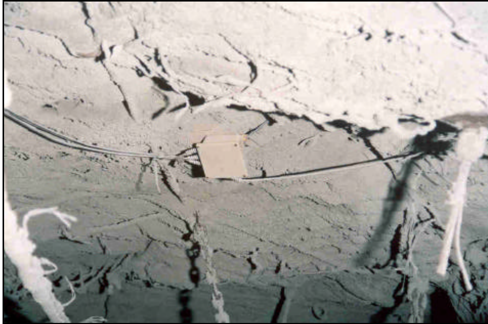
Figure 5.9. Close-up of the hangingwall condition adjacent to position 3.
