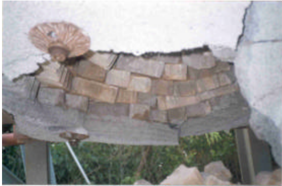
Figure A.45. Final failure of shotcreted assembly.
