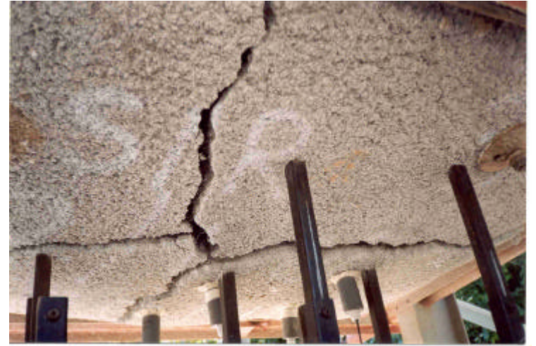
Figure A.43. Shotcrete 50 cm. drops.
