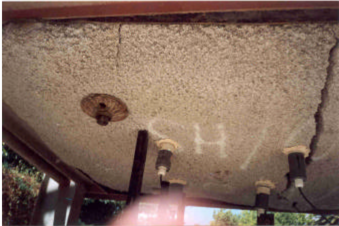
Figure A.42. Shotcrete 50 cm. drops.
