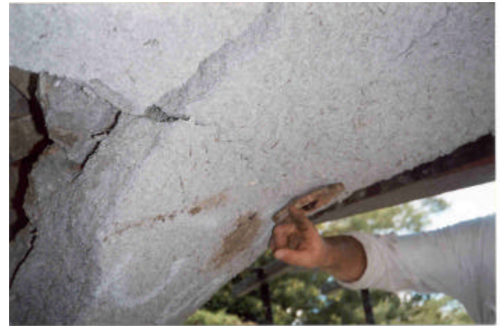
Figure A.44. Shotcrete 50 cm. drops.
