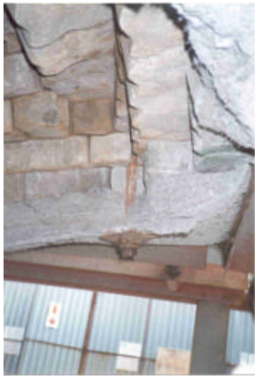
Figure A.46. Final failure of shotcreted assembly.
