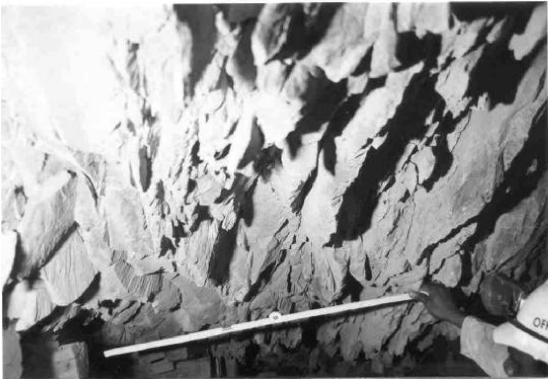
Figure 4.4.4 Hangingwall at middle of E1 panel, 94-48 VCR stope at Mponeng mine (face at left)
