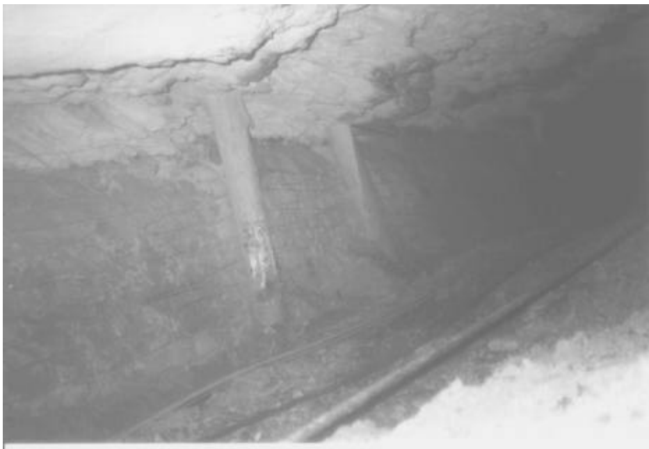
Figure 4.1.3 Rough hangingwall conditions in a backfilled stope at Kopanang mine
