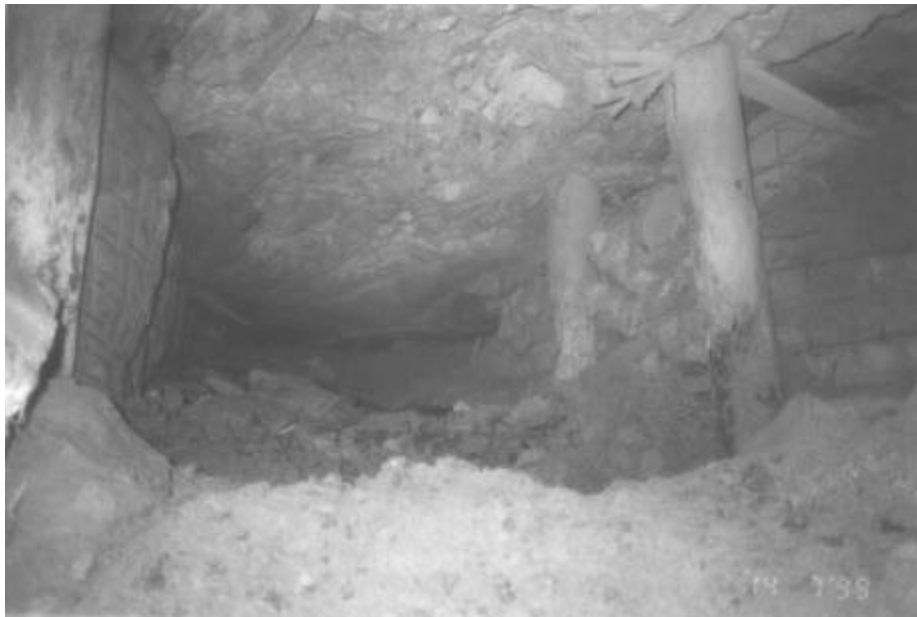
Figure 4.1.4 Variability of backfill placement at Kopanang mine, e.g. 1.5 m-wide gap left between backfill
