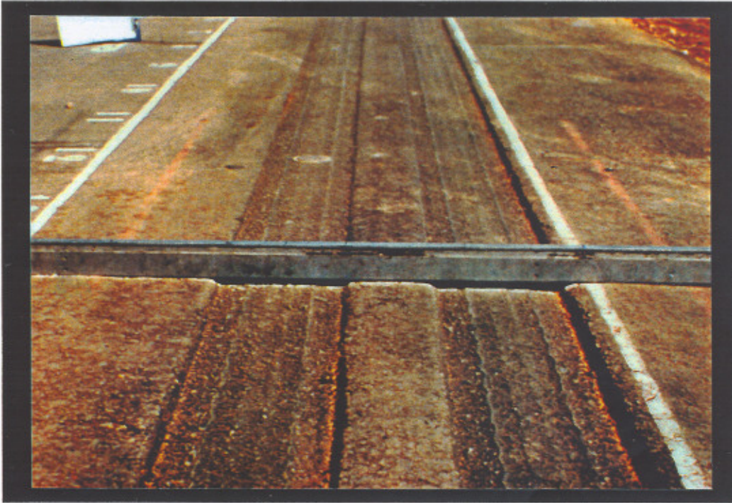
PHOTOGRAPH 5 : Rutting after channelized traffic
