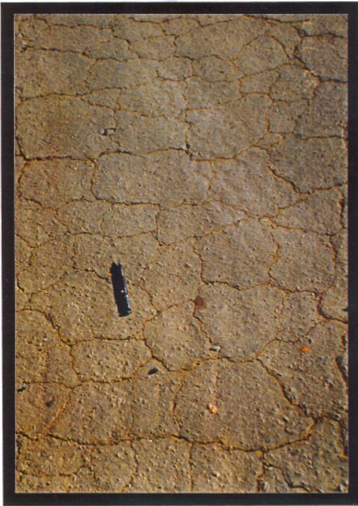
PHOTOGRAPH 1 : The surface of P6/1, Bapsfontein to Bronkhorspruit currently showing extensive cracking _
