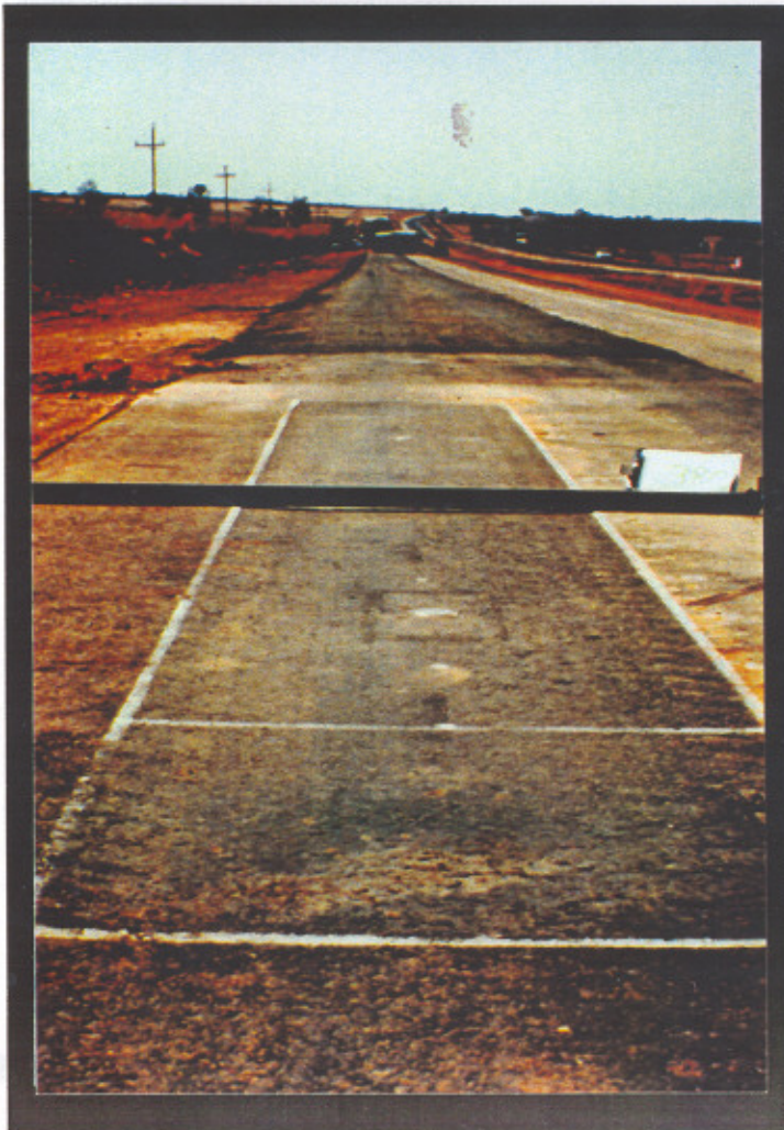
PHOTOGRAPH 6 : Rutting after wandering traffic
