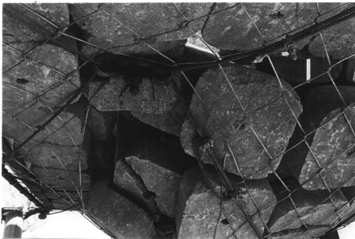
b) S-W corner; approx. 380 mm of yield occurred at loop clamped with 2 Crosby clamps tightened to 15 Nm.
