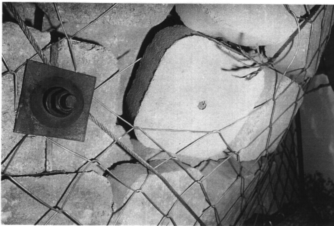
a) The 8 mm lacing failed at the N-W face plate on one diagonal.
