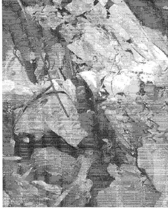
Figure B.23 View south along 24-26 haulage east at end of area of hangingwall collapse showing the highly fractured nature of the immediate hangingwall rock mass, and remaining rock bolt reinforcement.
