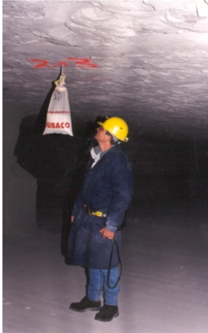
Figure 5.1b: Stone dust bag suspended in the mine entry
