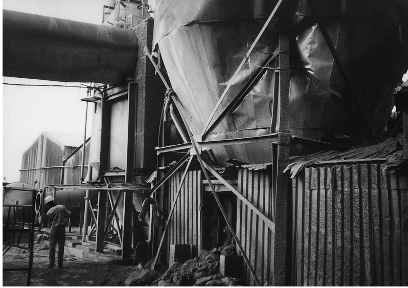
Fig. 1. View of base of collapsed drier.
