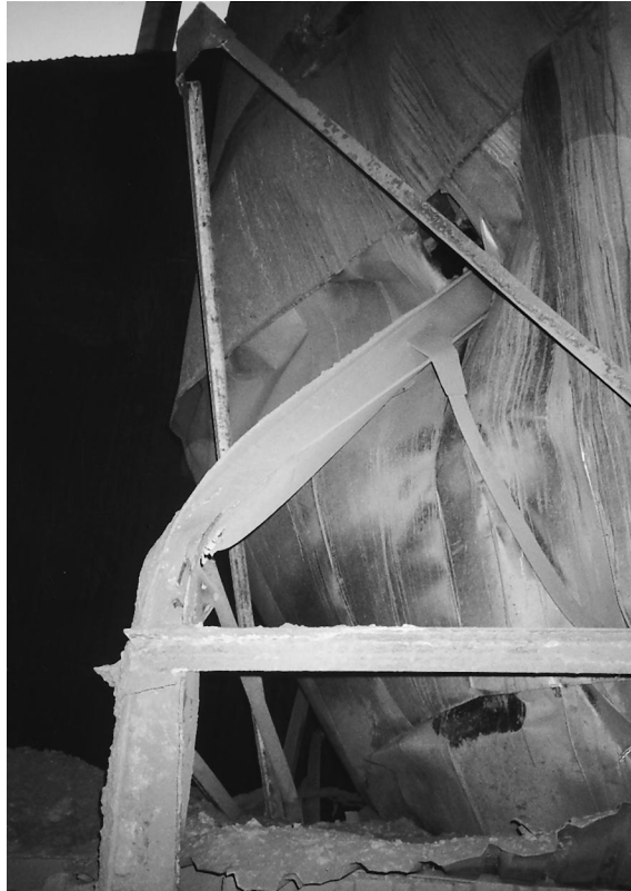
Fig. 3. View of buckled column.
