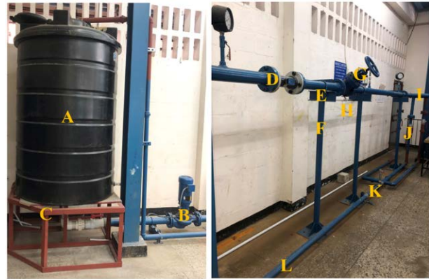
Figure 1. Components of the experimental piping system
