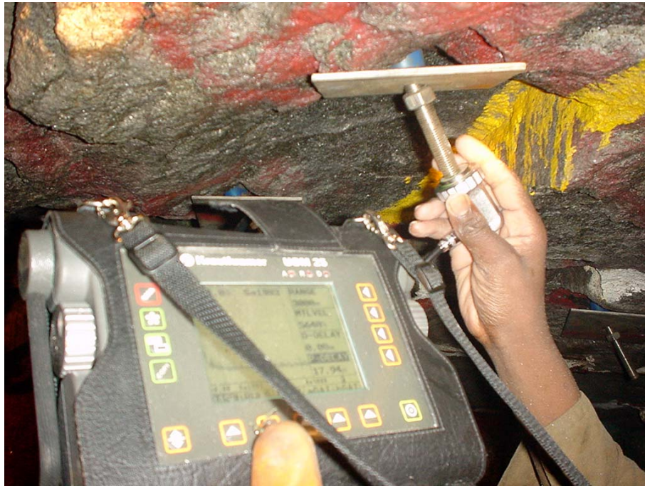
Figure 23. Monitoring of a smartbolt (with a flat base plate) using an ultrasonic device
