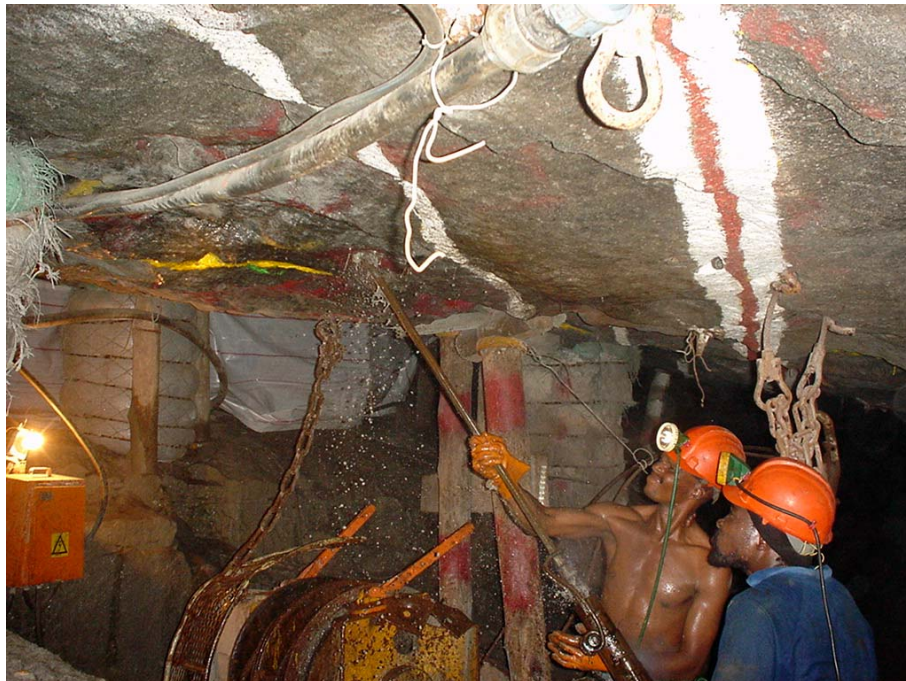
Figure 22. The drilling stage prior to installation of the required roofbolt at a platinum mine test site
